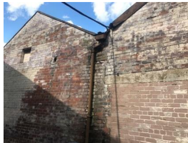
Stained brick walls – leaks from valley gutters / defective fall pipes and hoppers
