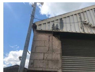
Cracking and peeling
