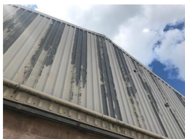
Peeling plastisol sheeting
