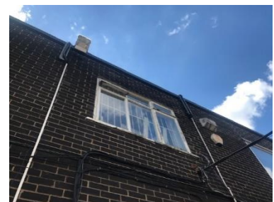
Deteriorating timber window
