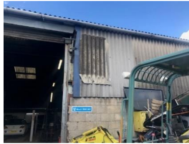
Broken asbestos sheeting
