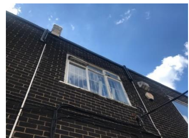
Deteriorating timber window
