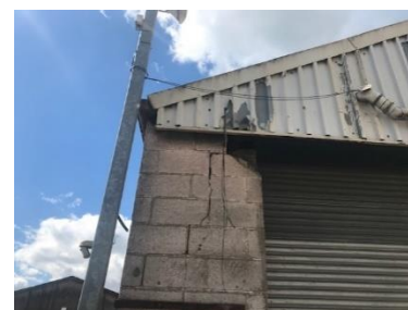
Cracking and peeling
