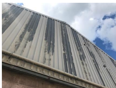
Peeling plastisol sheeting
