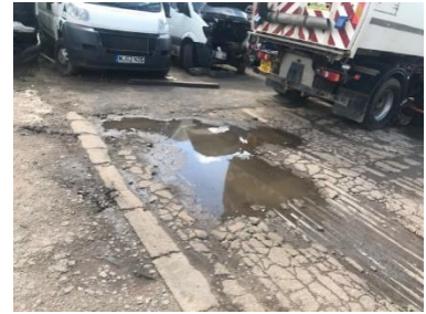
Deteriorating yard areas
