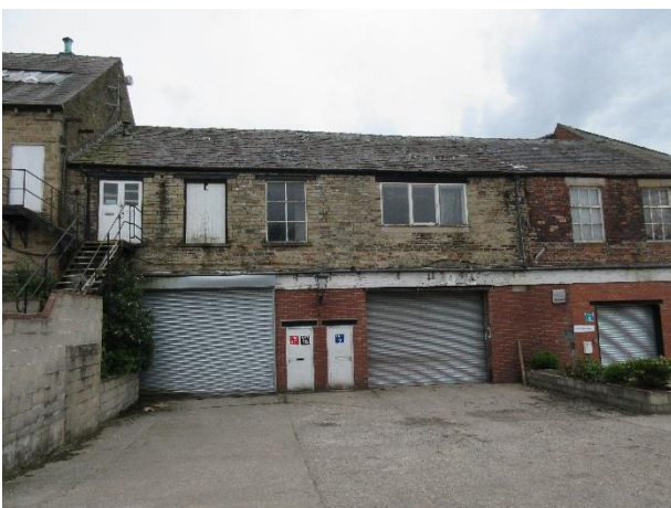
Units 25 and 25B
